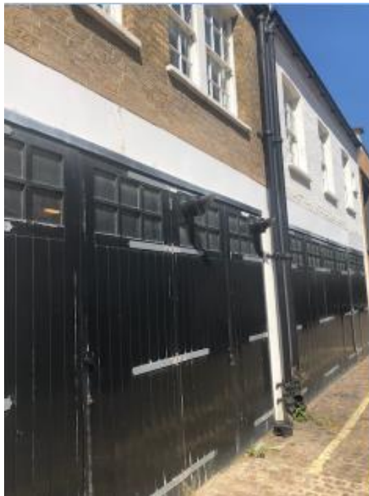
Detailed view of the flues as Installed
